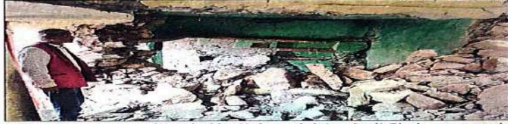
In Nov 2023, a committee led by Union minister Amit Shah, approved a recovery plan worth Rs 1,658 crore for subsidence-hit Jyotirmath
