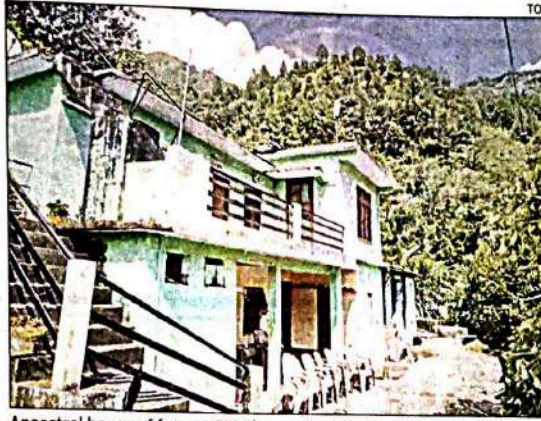
Ancestral house of former CM Bhagat Singh Koshyari has also been impacted as the courtyard wall has begun to tilt precariously
